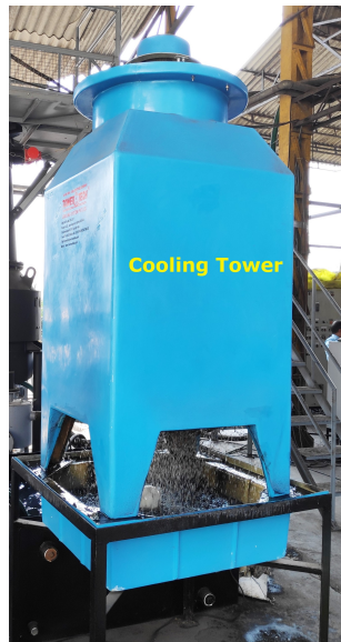
(a) Cooling Tower
